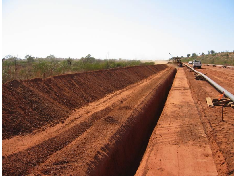
Plate 1: Open Trench with Strung Pipe on Right and Lowering in Machine at Rear
